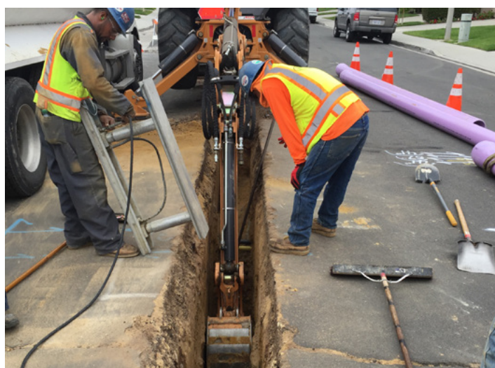
MNWD's Recycled Water System Extension Project provided over 33 million gallons of recycled water a year to 12 new recycled water services in the Laguna Audubon HOA and 20 other recycled water services in the Cities of Aliso Viejo, Laguna Hills, and Laguna Niguel, as well as recycled water pipelines in Aliso Viejo, Laguna Hills, and Laguna Niguel.
